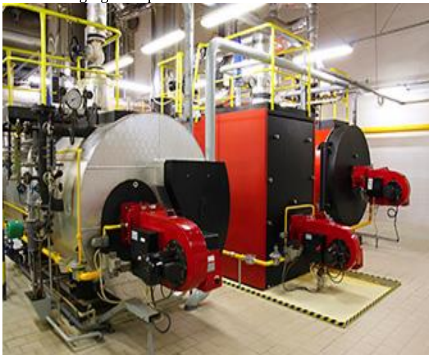
Fig.2. 4. A stationary boiler
